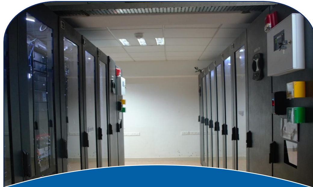
State-of-the-Art Data Centre
